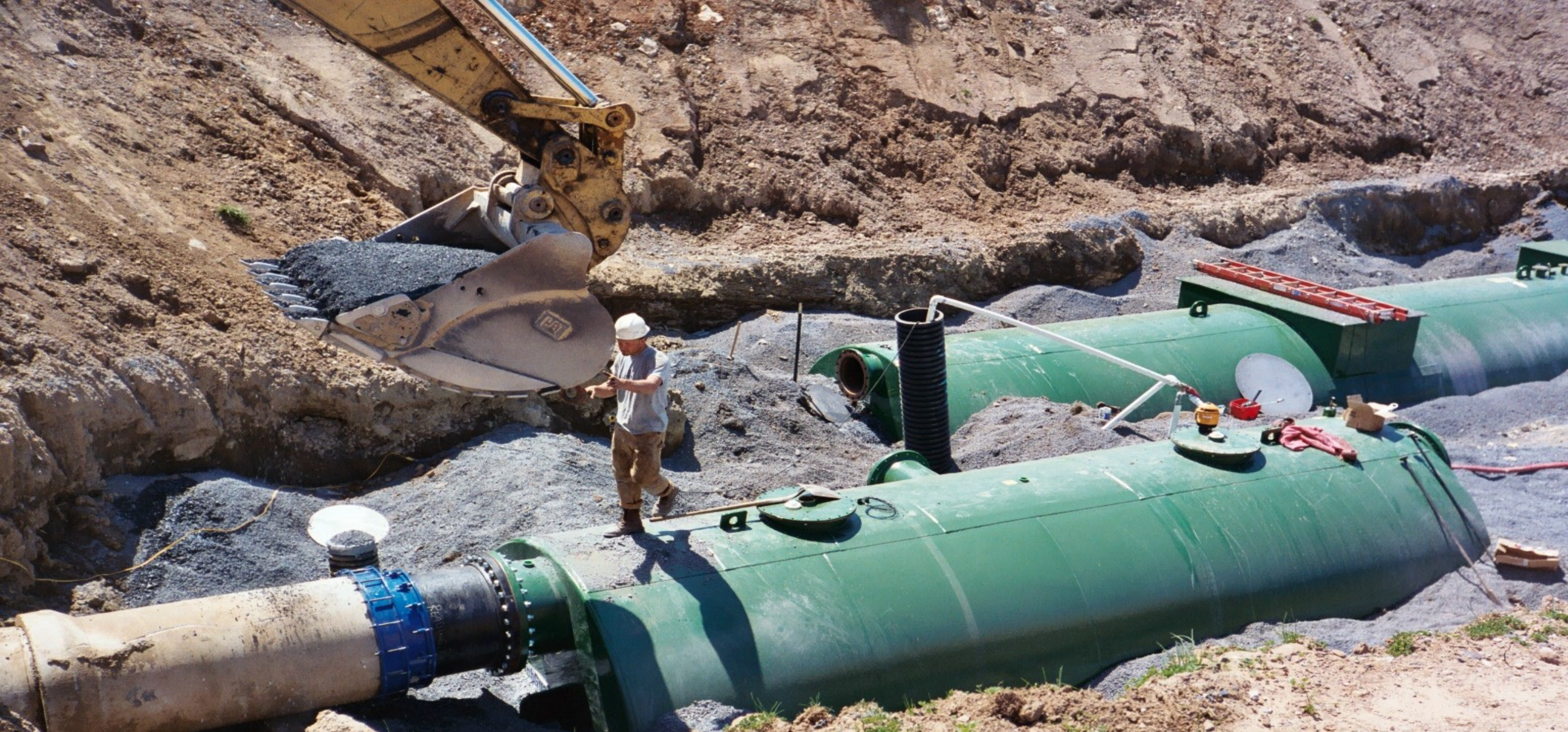
(1) 15,000 INTERCEPTOR/30,000 OWS STORMWATER MANAGEMENT SYSTEM AT AIRPORT RUNWAY
