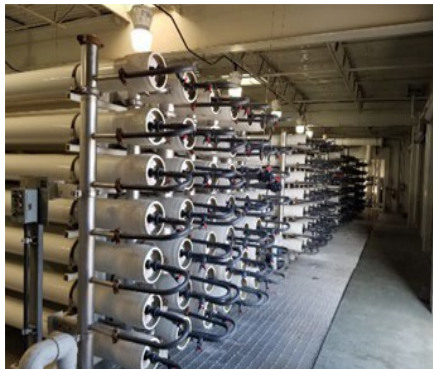
Membrane (Reverse Osmosis or Nanofiltration)
